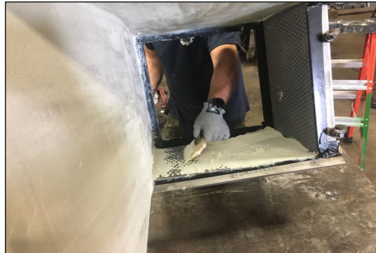
In process: ARC MX FG being applied to prepared and tack welded surface.
