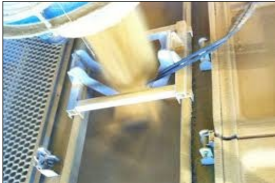
Before: chute in service.
